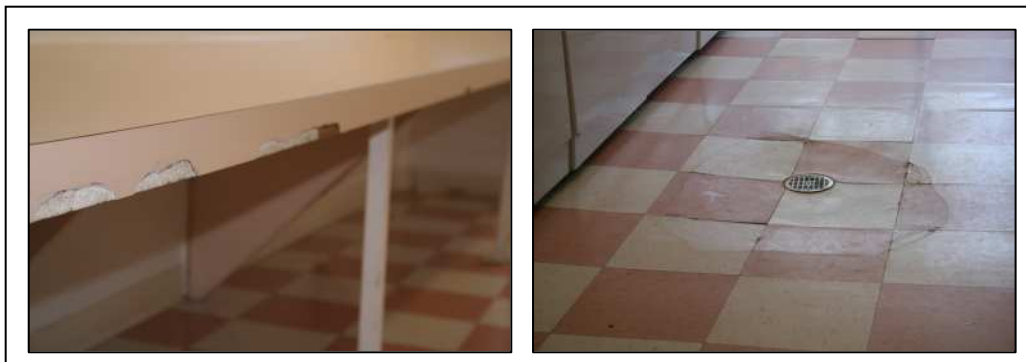
Prior to renovations, the Season's laundry rooms showed signs of disrepair common in many communities that contribute to the negative perception of central laundry in the industry.
